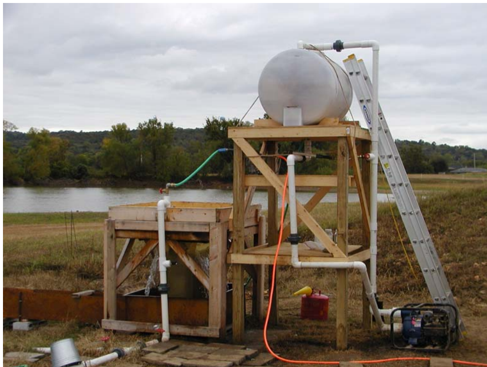
Figure 2. Side view of pilot scale set up.
